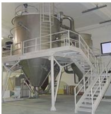
Figure 1 – Spray dryer installations at IEN
